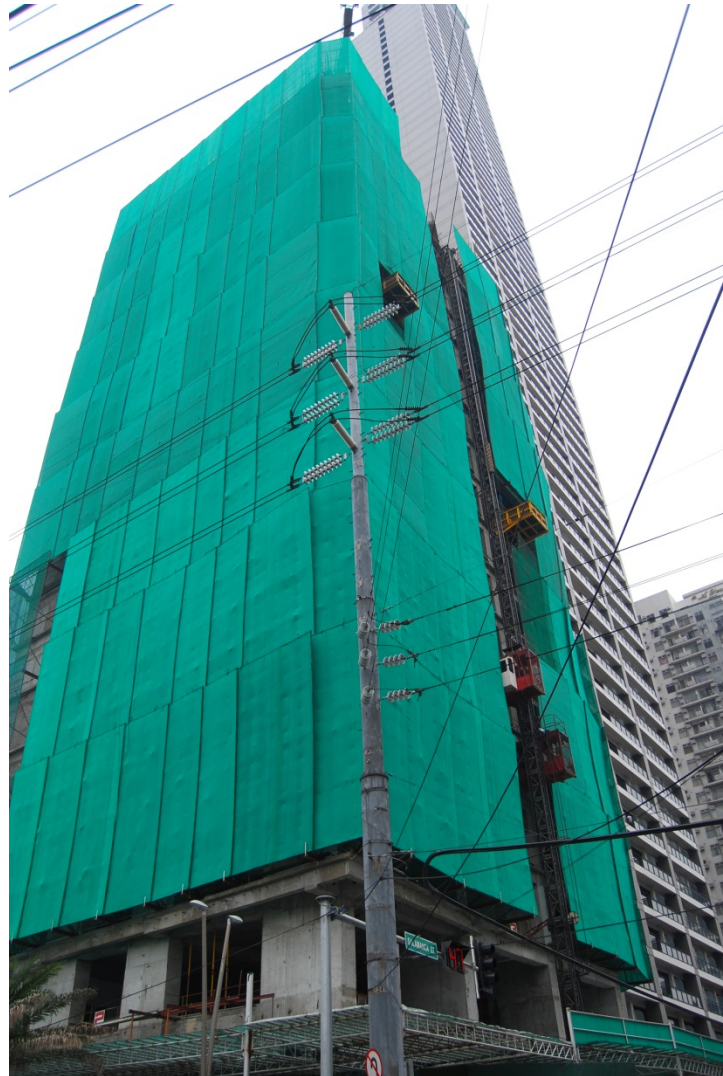
Trump Tower at Century City is on its 22 nd level this month.
