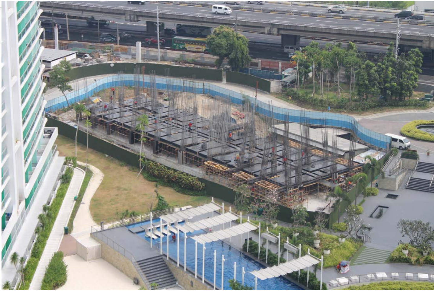
Boracay Tower now stands at 2 floors and is currently undergoing structural formworks .
